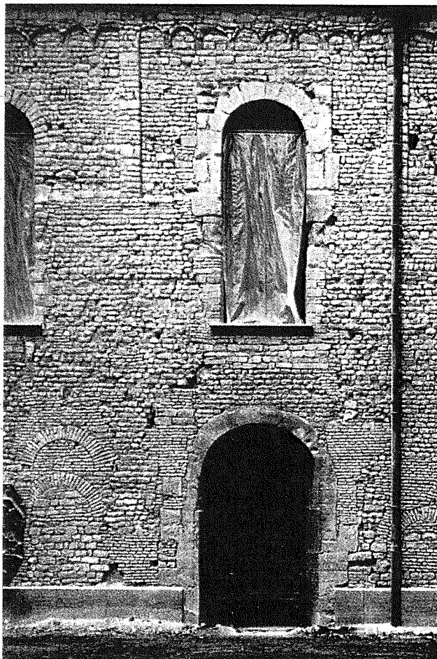
FIGURE 1. Speyer, Cathedral of St. Mary and St. Stephen. Construction of the outer walls in the nave (courtesy of the Zentralinstitut für Kunstgeschichte, Munich).
